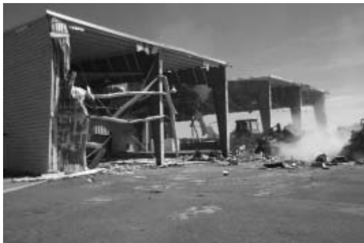
Old hangars are cleared from the site for the new, 90,000 sq.ft. facility of Signature Flight Support.
